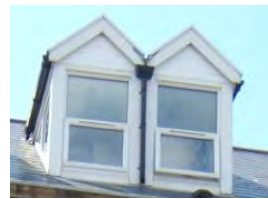
Inappropriate dormers in the 19th/early 20 th Century Terraces Sub-Area
